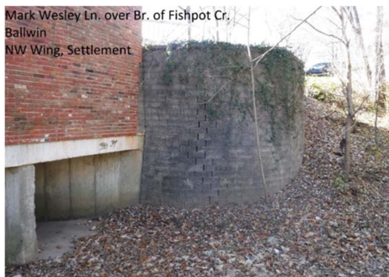
Smith Drive Culvert recommended for replacement
